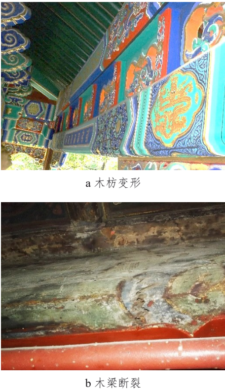
图3 木构件的竖向变形及断裂 Fig.3 Vertical deformation and fracture of wooden components
